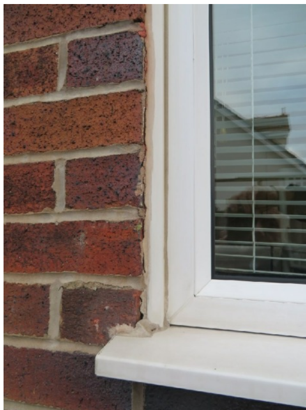
Shrunken seals around window frames
