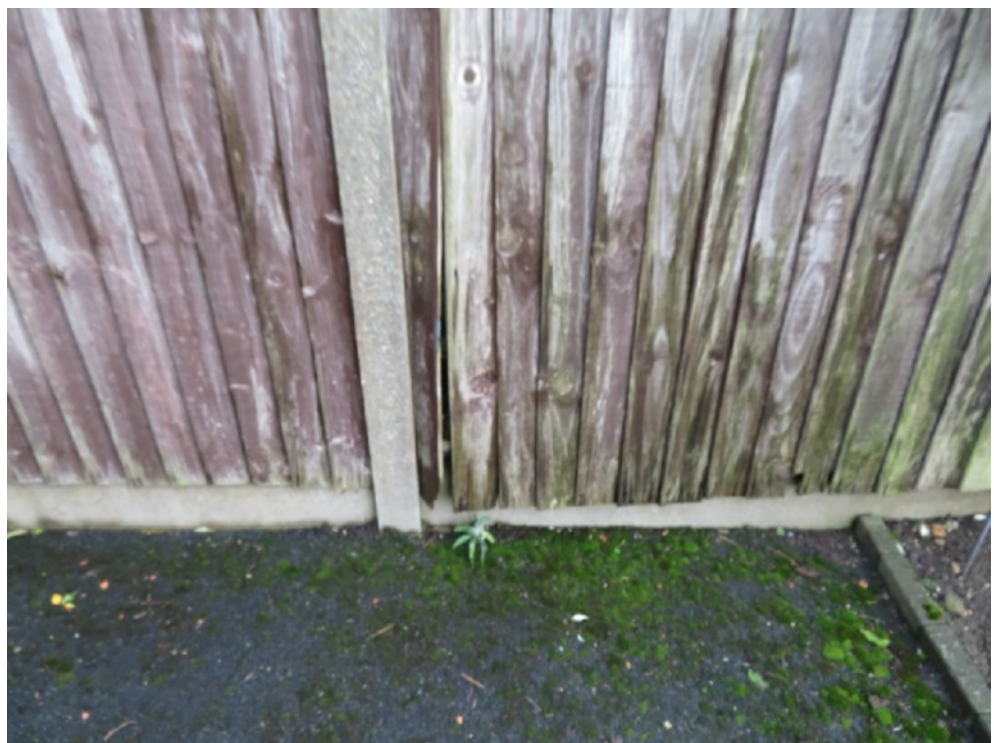
Rot to fence
