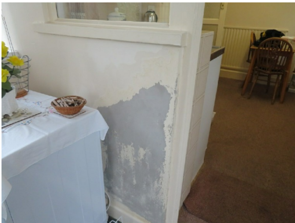
Damp stained wall in sun room
