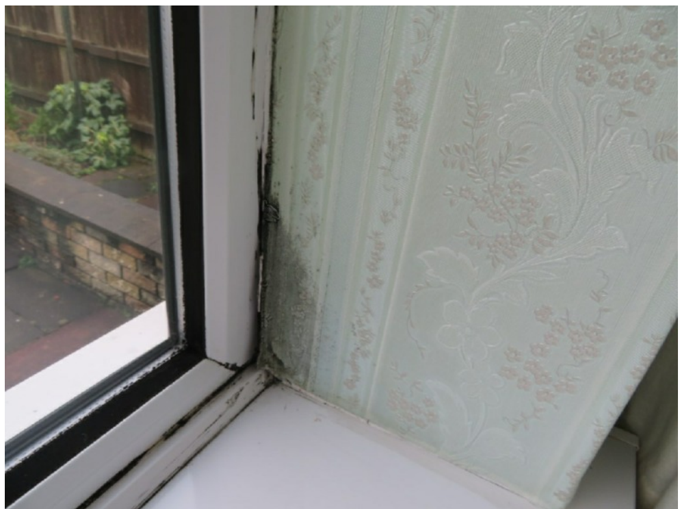
Damp stained window reveal
