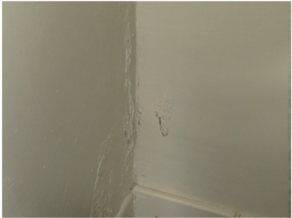
Damp stained wall in sun room
