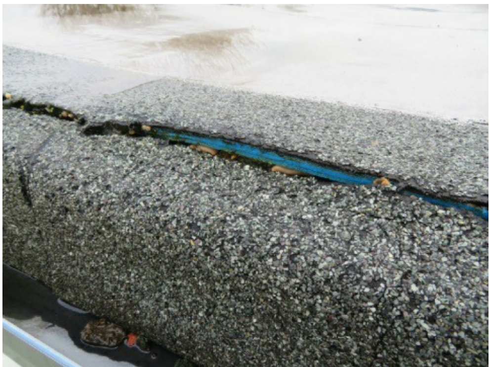
Collapsing flat roof
