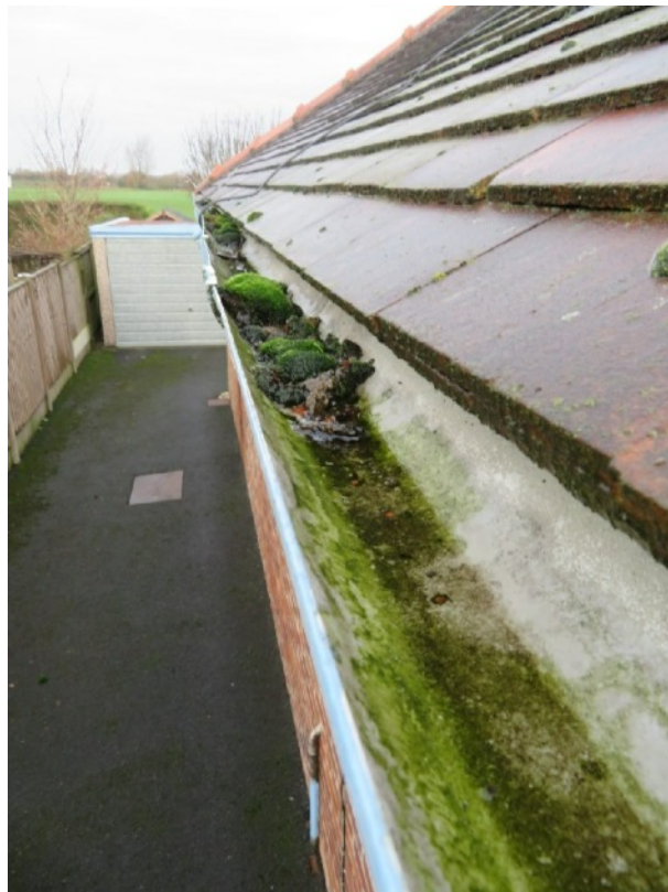
Moss and silt in gutter
