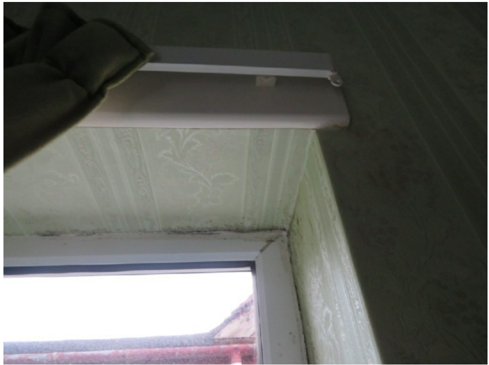
Damp stained window reveal
