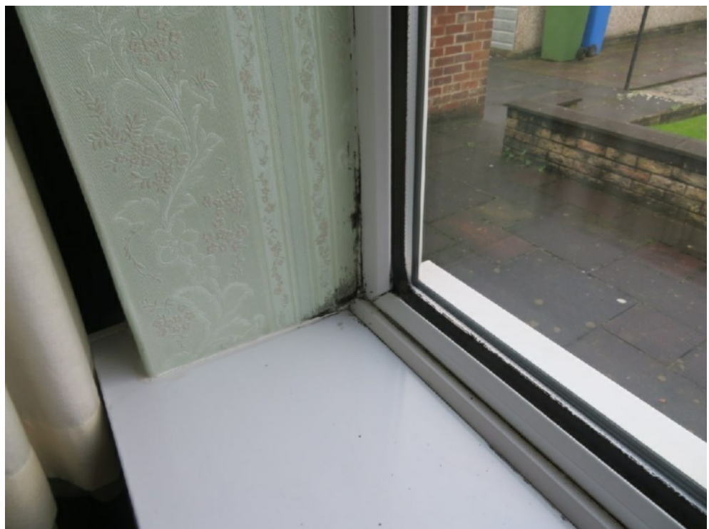
Damp stained window reveal
