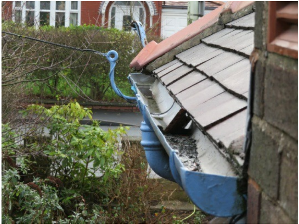
Debris in gutter
