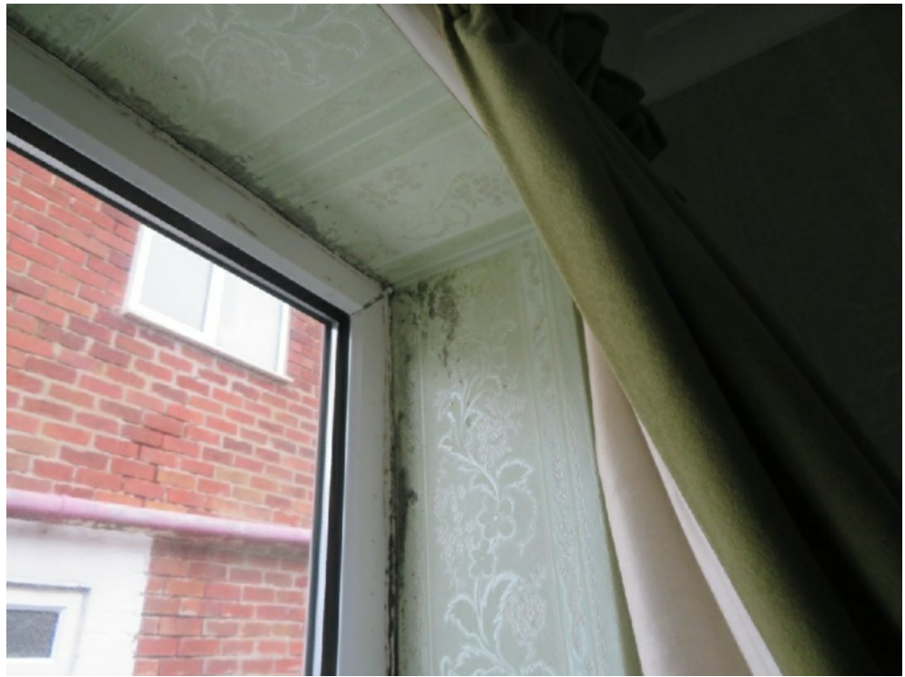
Damp stained window reveal
