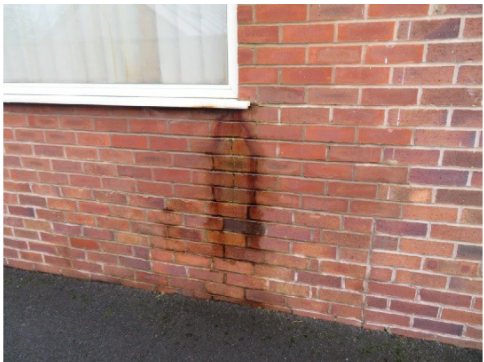
Damp staining to external wall below flat roof
