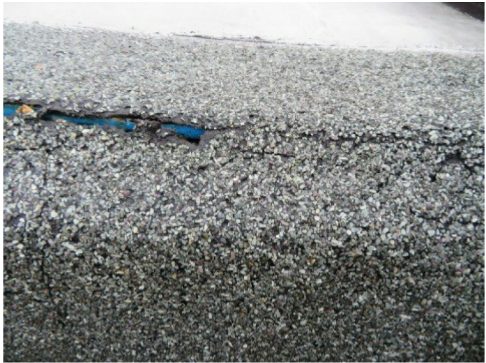
Collapsing flat roof
