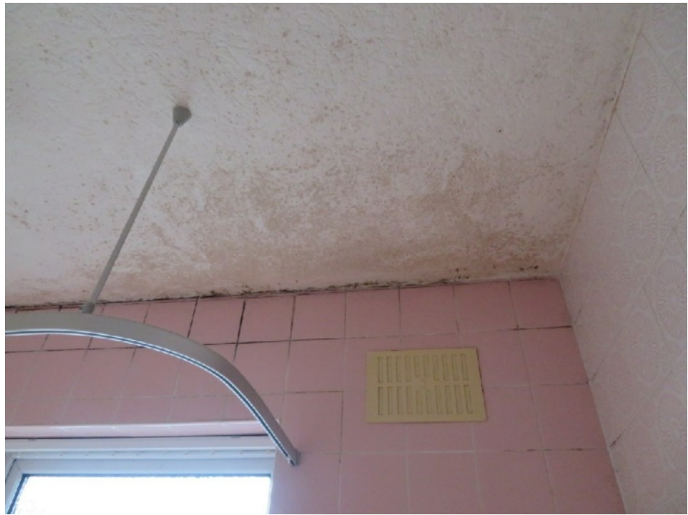
Damp stained ceiling in bathroom
