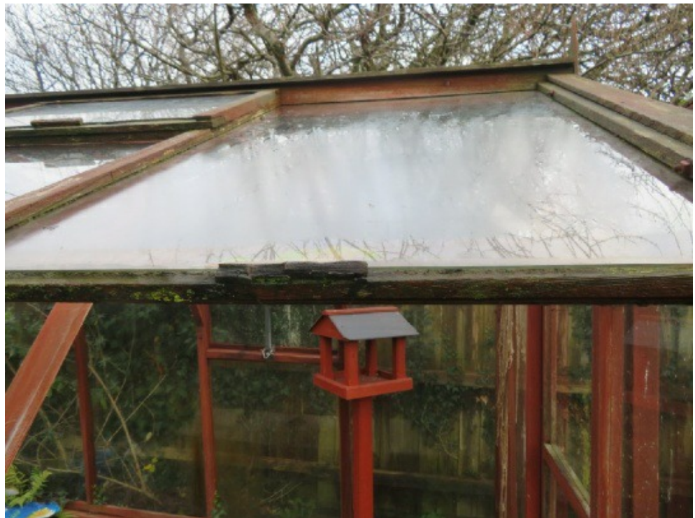
Rot to glass support on greenhouse
