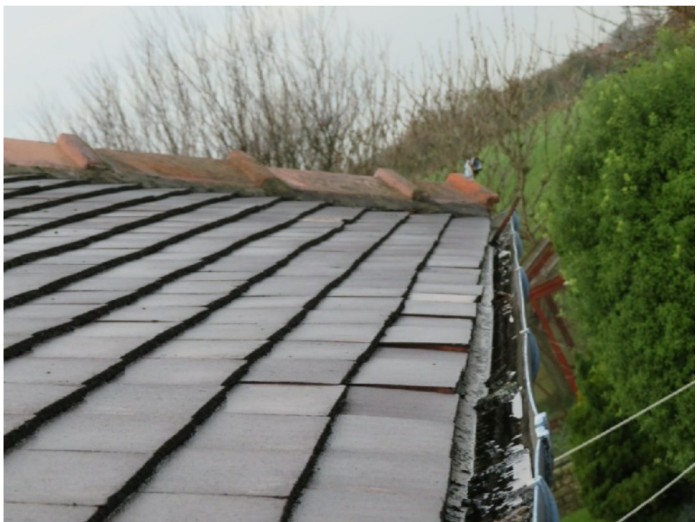
Moss and silt in gutter
