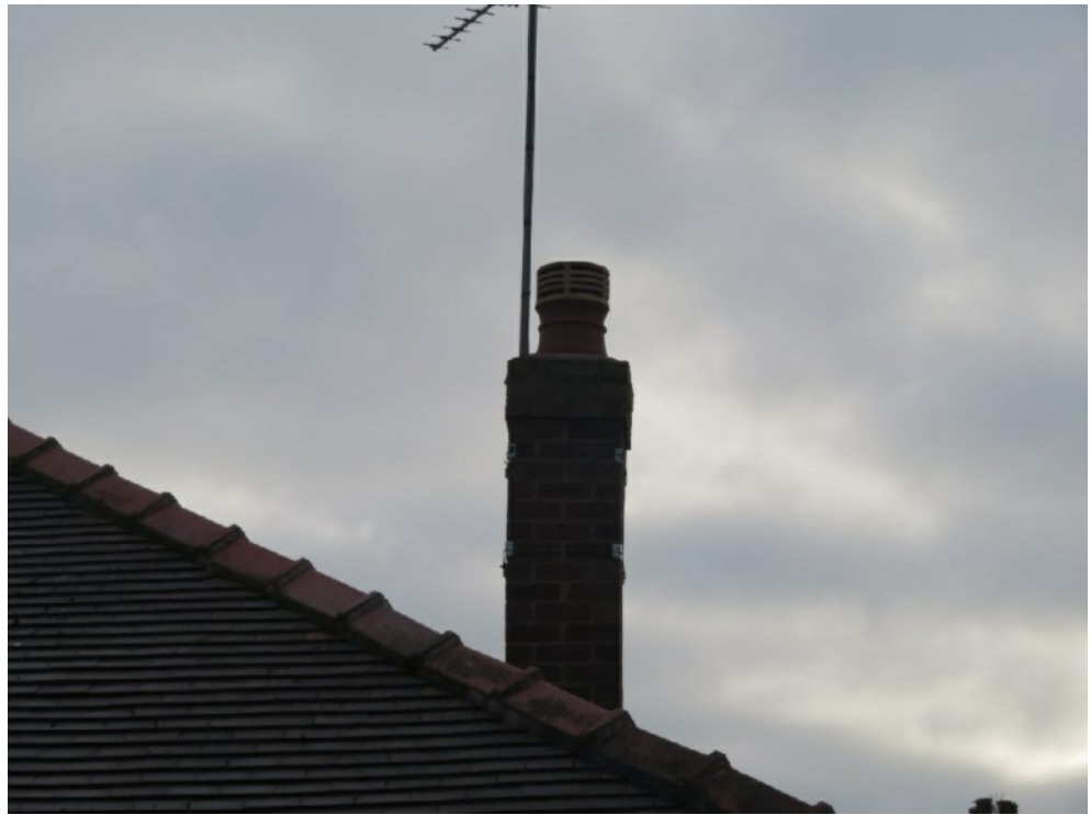
Slight lean to chimney stack
