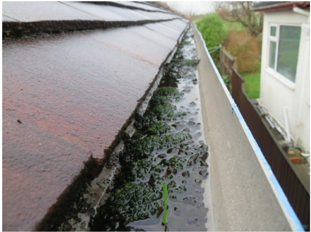
Moss and silt in gutter
