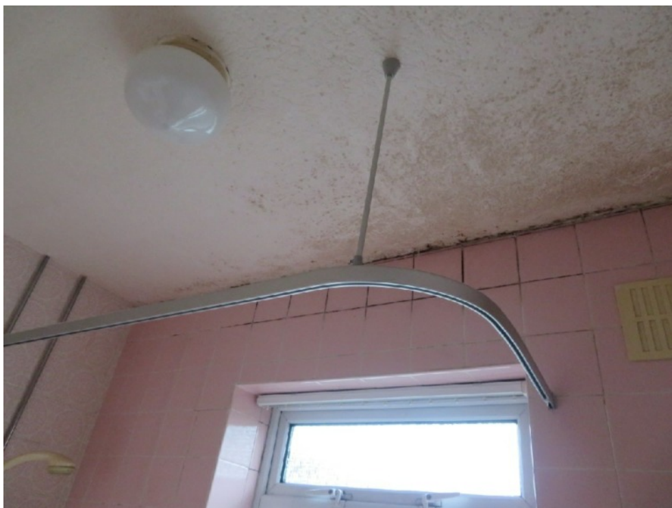
Damp stained ceiling in bathroom
