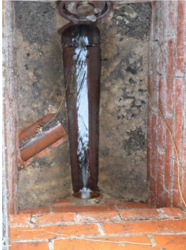
Roots in drains
