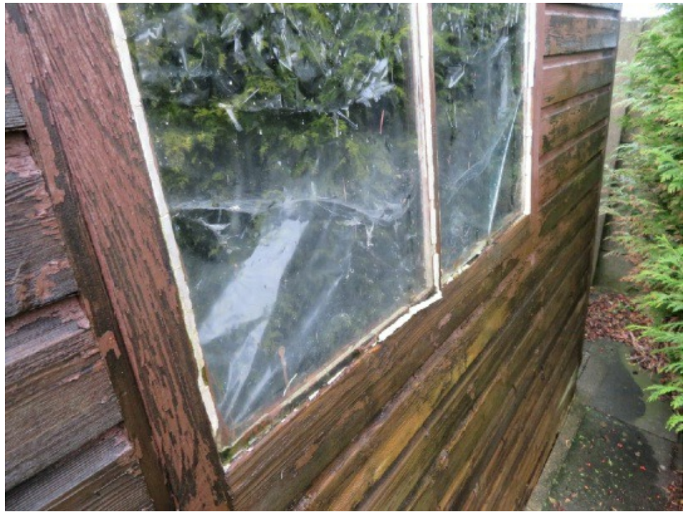
Rot to garden shed
