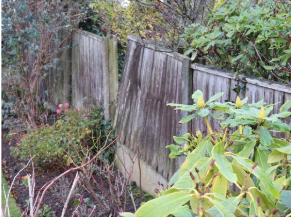
Loose fence panel
