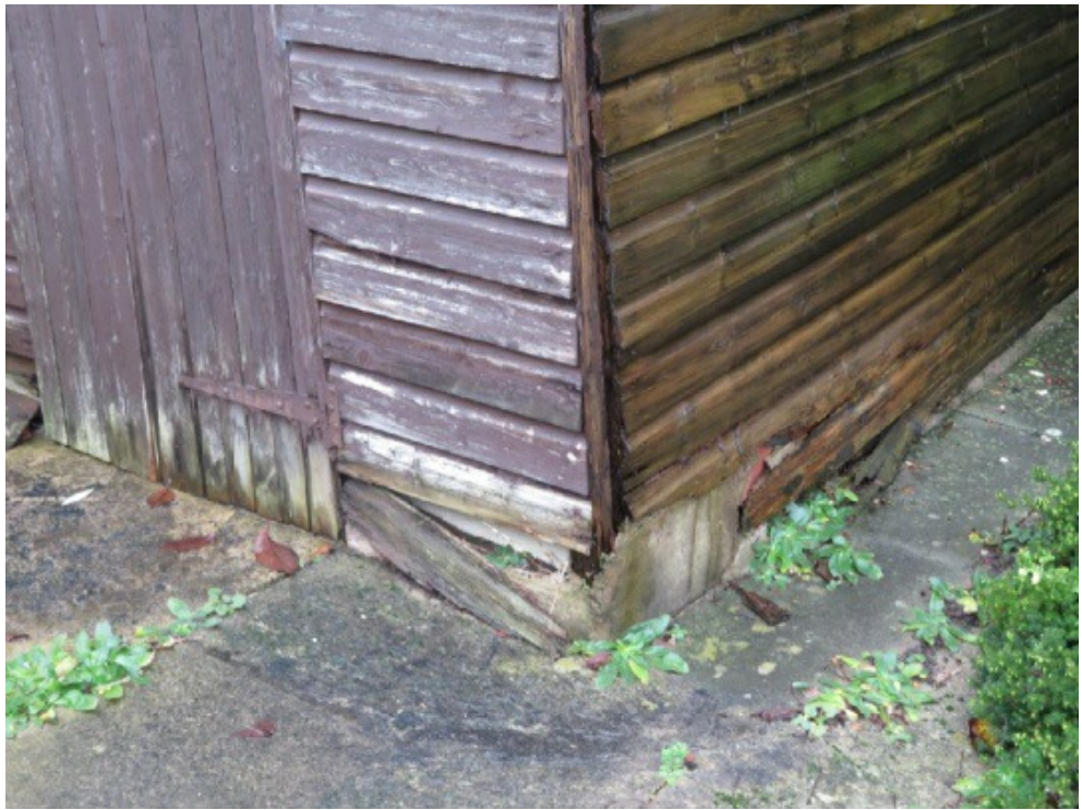
Rot to garden shed
