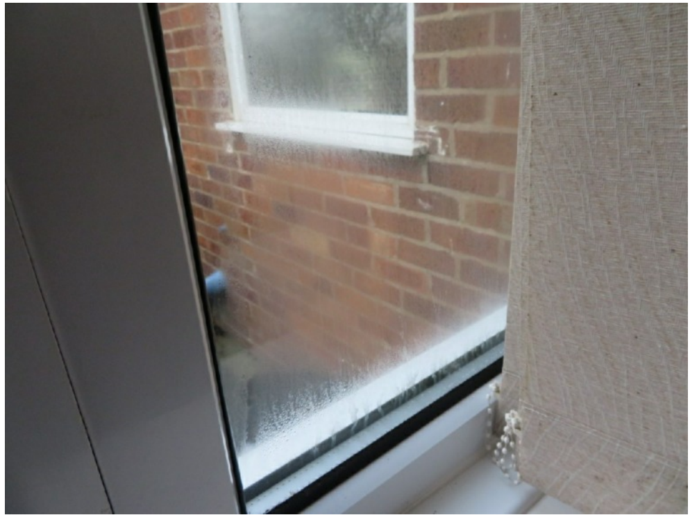
Misted window (failed seal)
