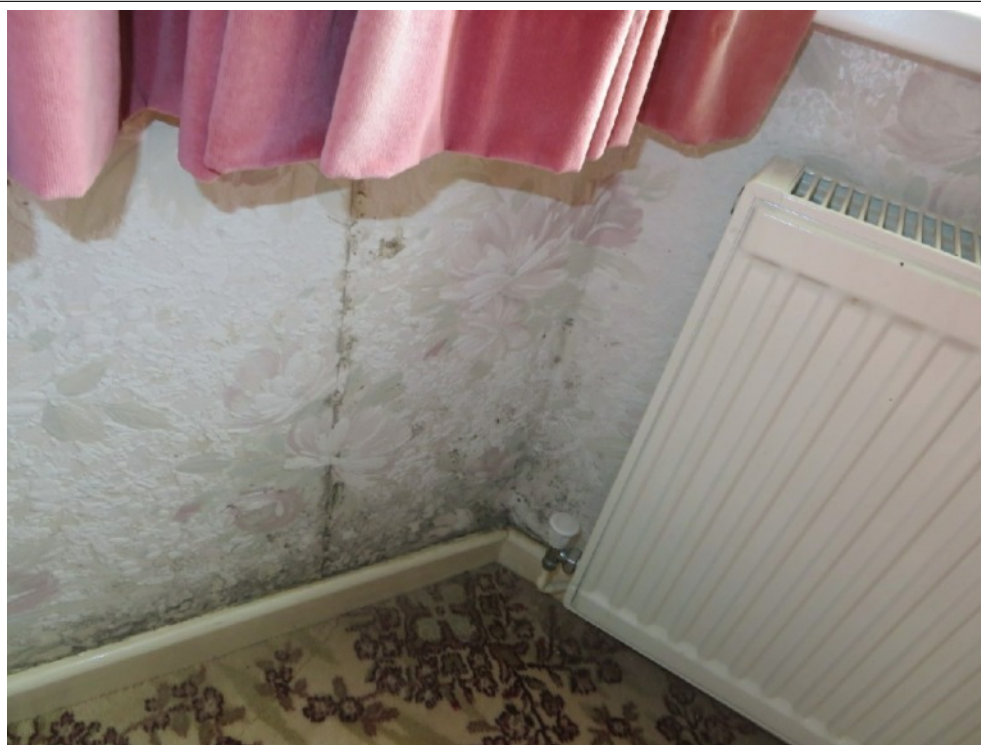
Damp stained wall in bedroom one
