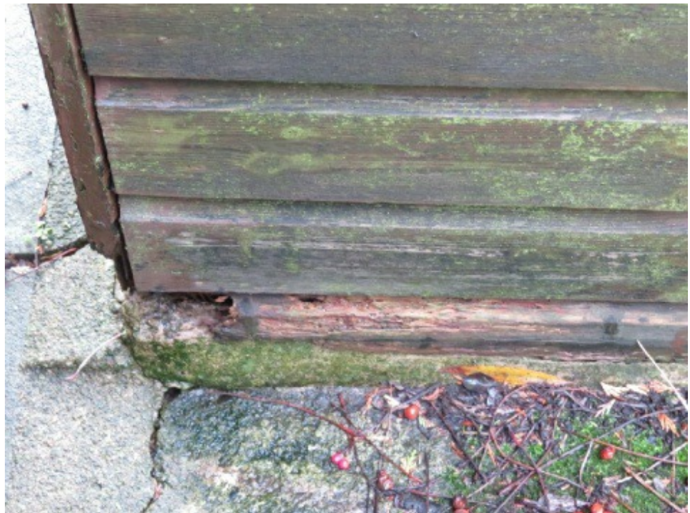
Rot to garden shed
