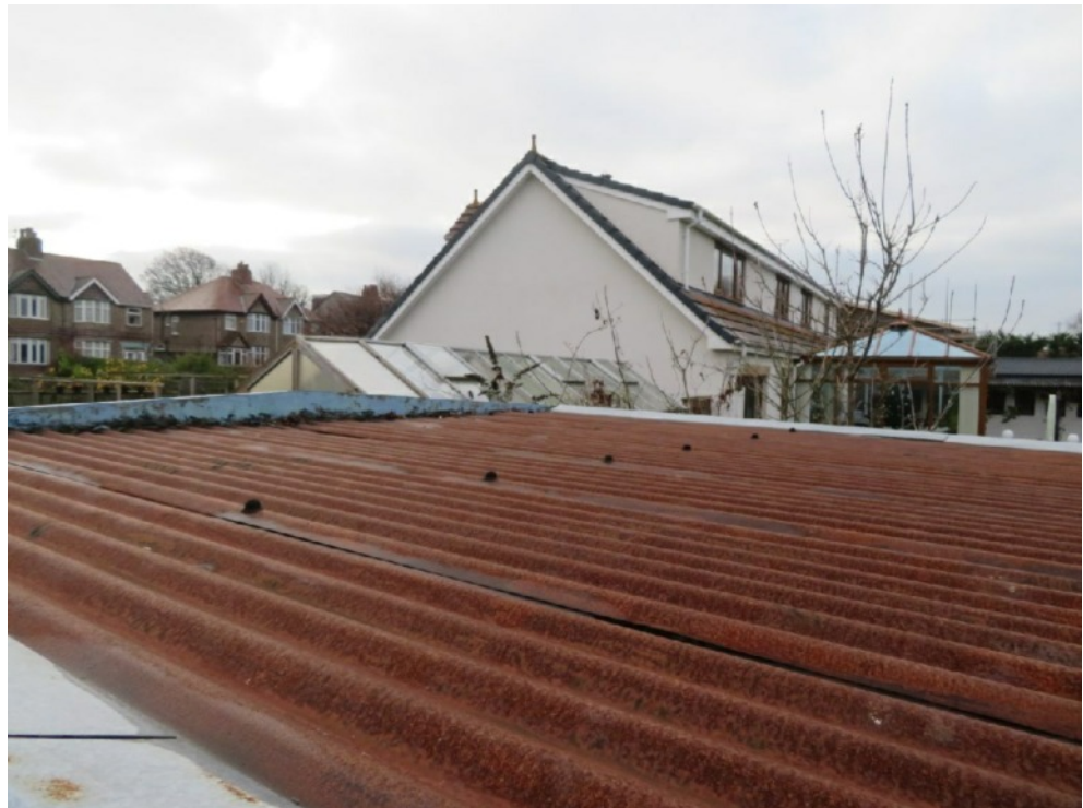
Rust to garage roof
