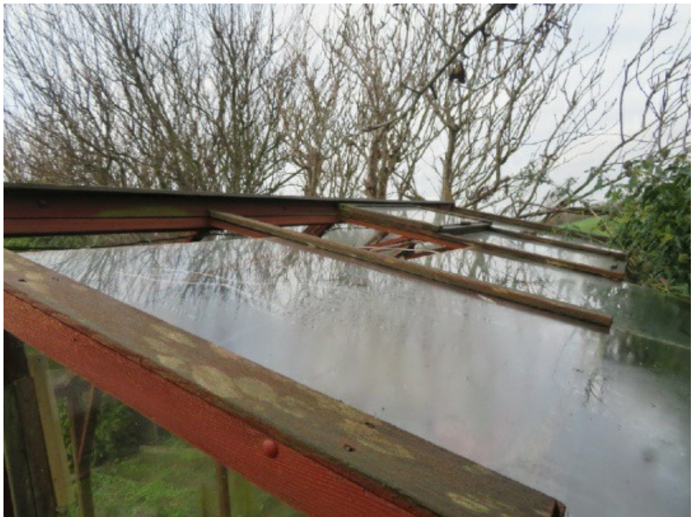
Loose glass to greenhouse
