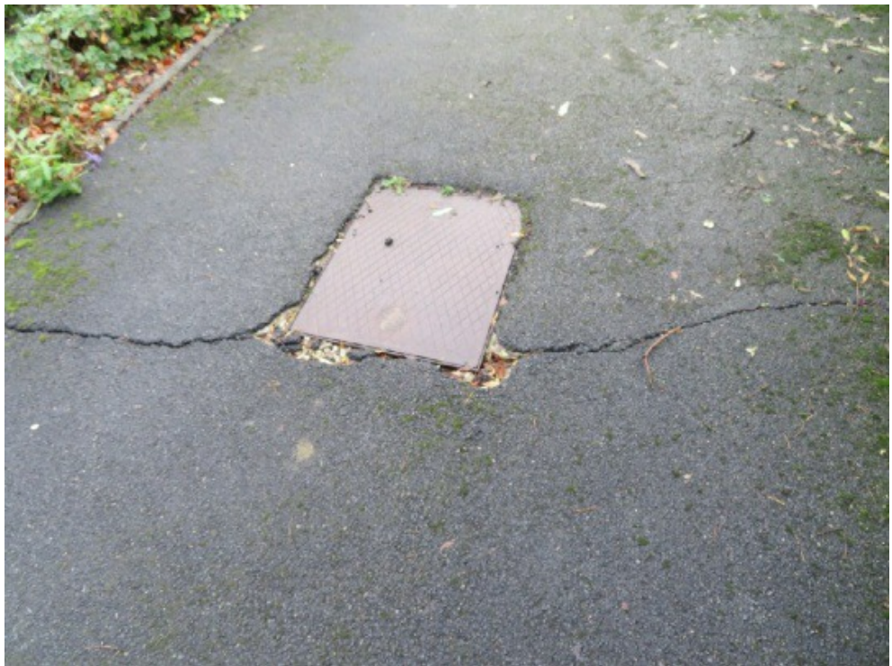
Crack to driveway
