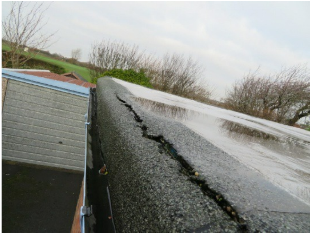
Collapsing flat roof
