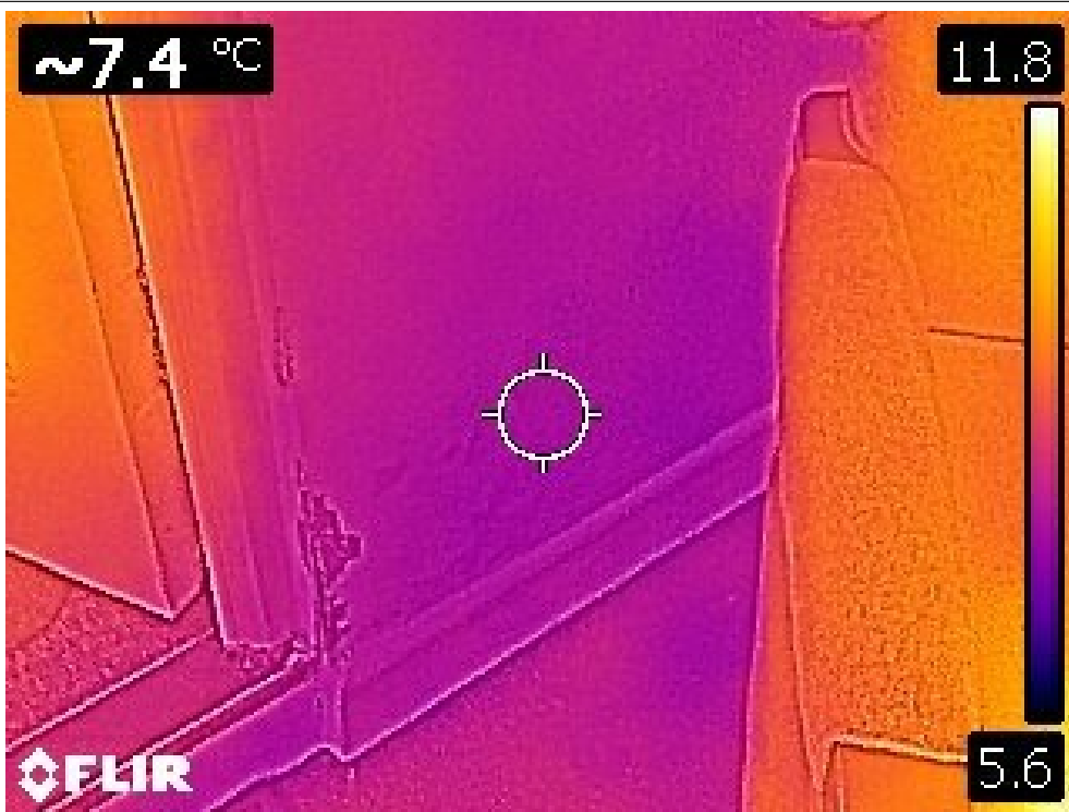
Thermal image of damp stained sunroom wall
