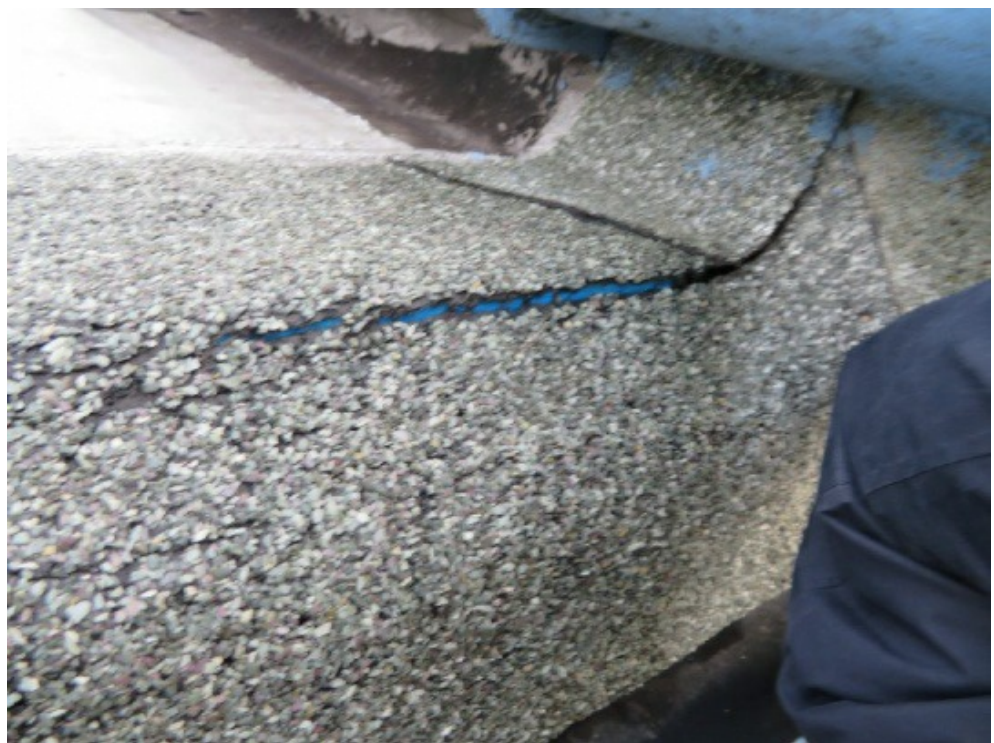
Collapsing flat roof
