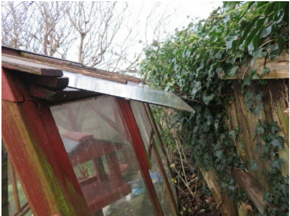
Loose glass to greenhouse
