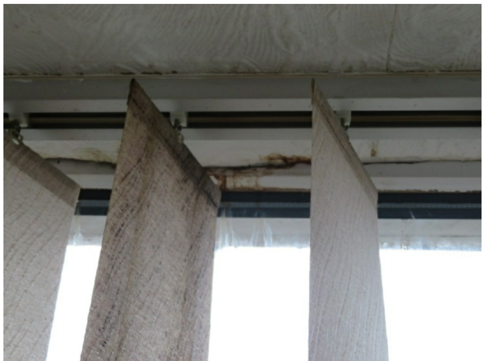
Leak from flat roof
