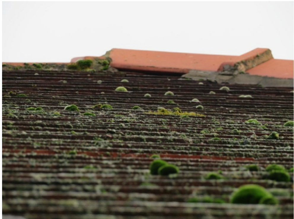
Moss to main roof
