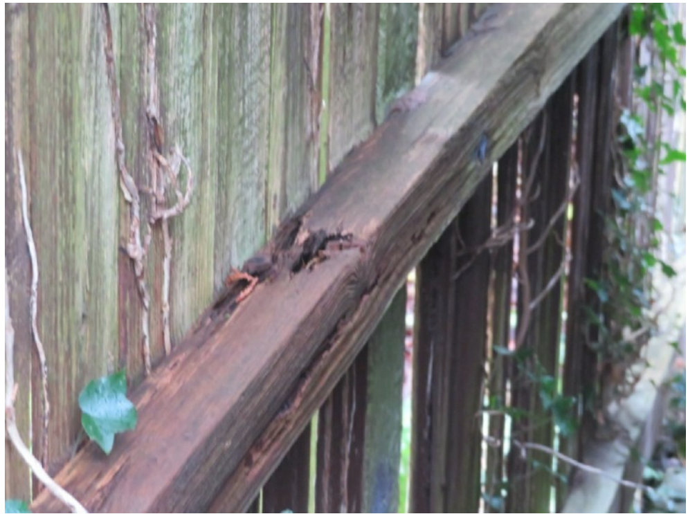
Rot to fence
