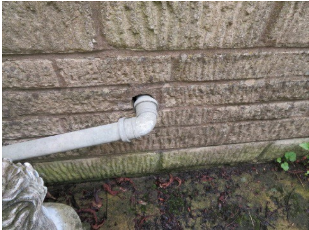
Gap around pipe at rear
