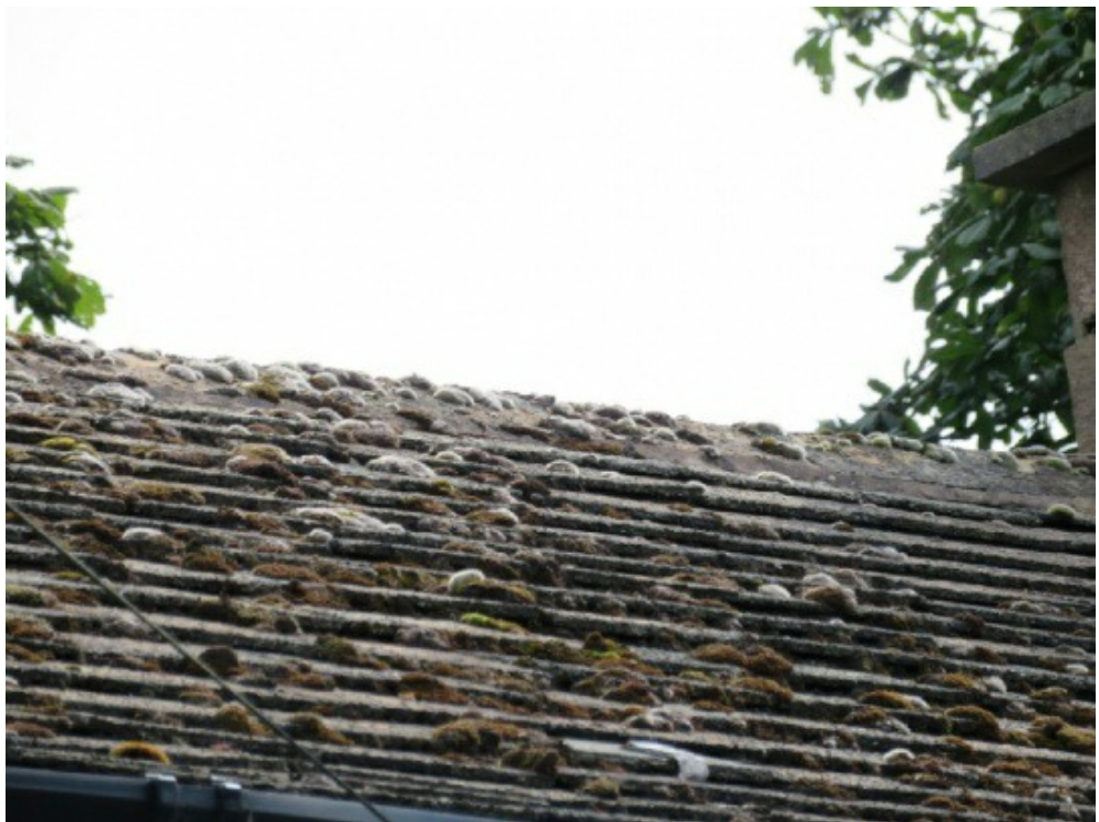
Moss on roof
