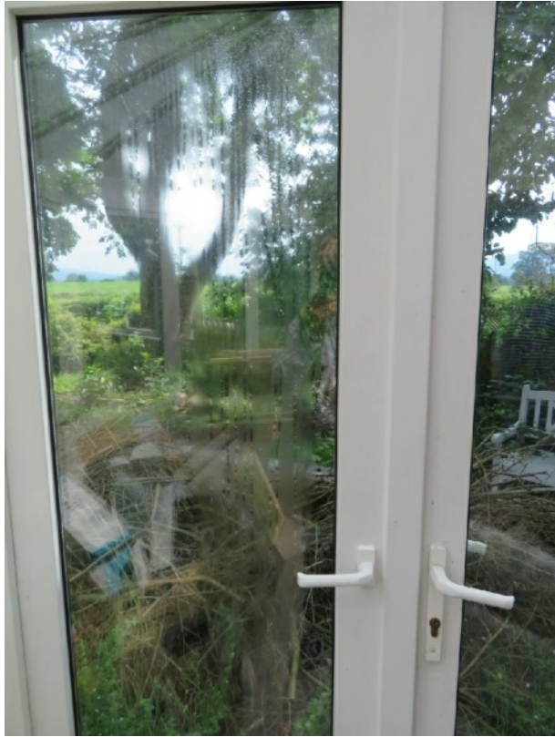
Misted (failed seal) window to conservatory
