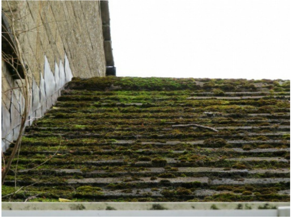
Moss on roof
