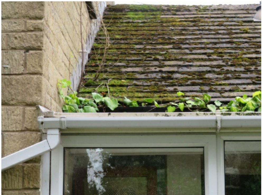
Tree growth on roof
