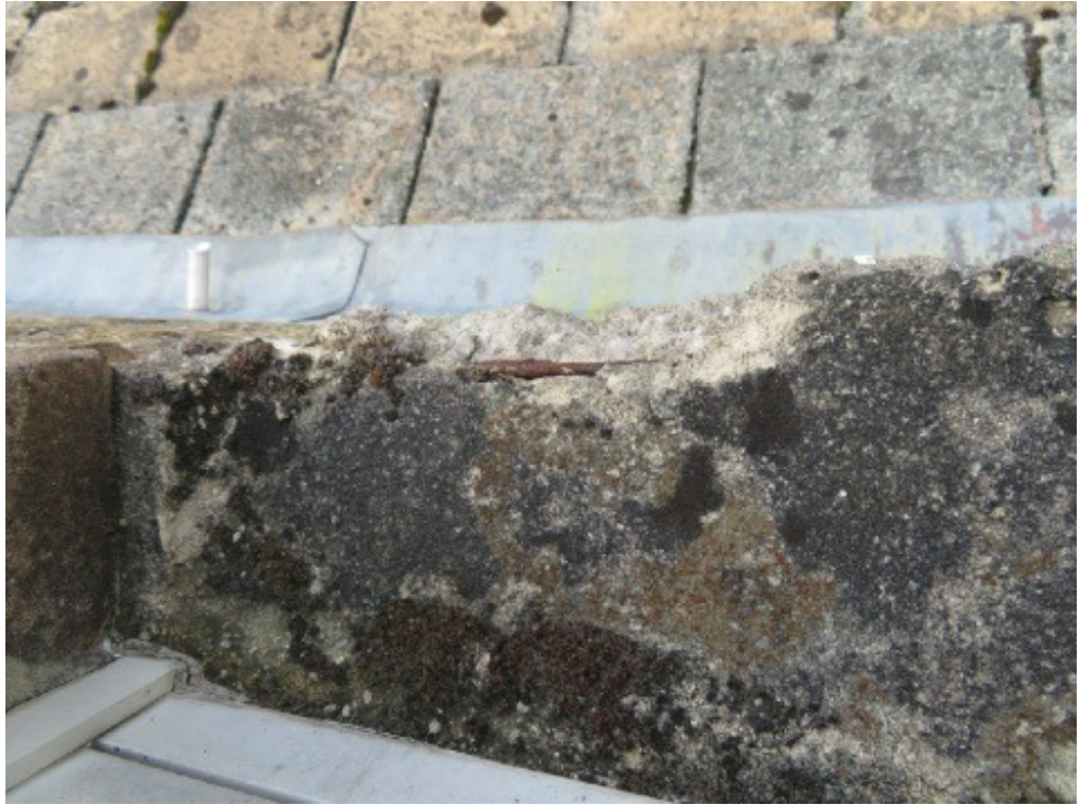
Spalled (frost damage) to window sill
