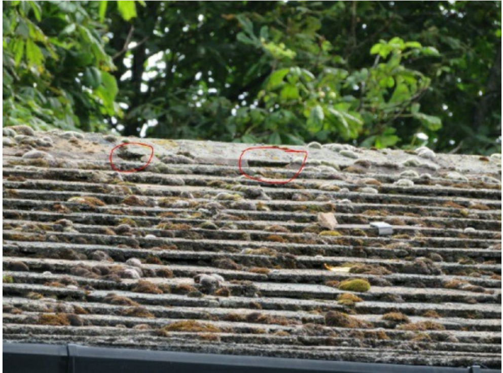
Incomplete mortar to ridge tiles
