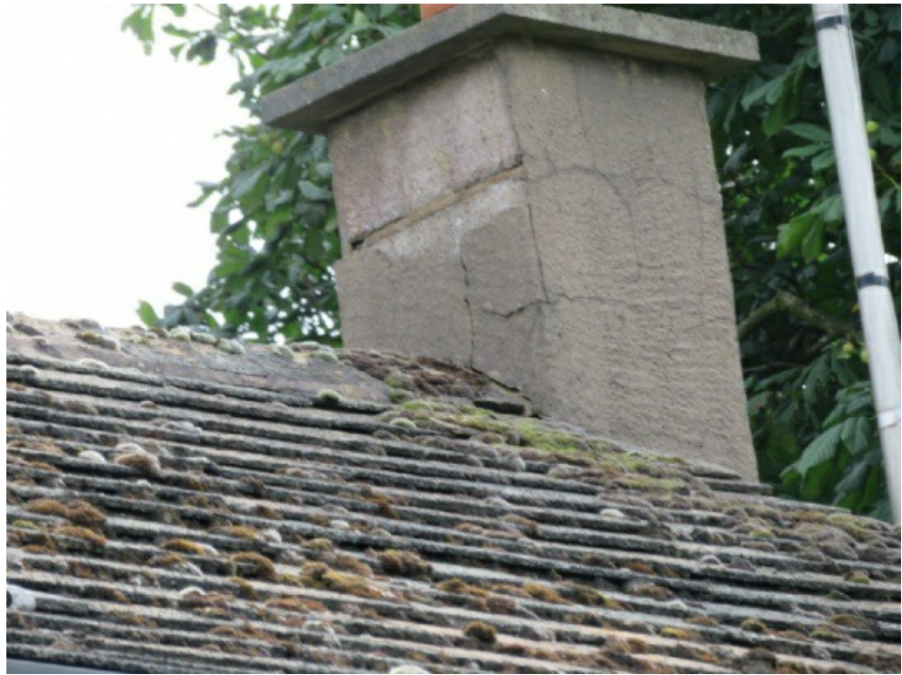
Cracked render to chimney stack
