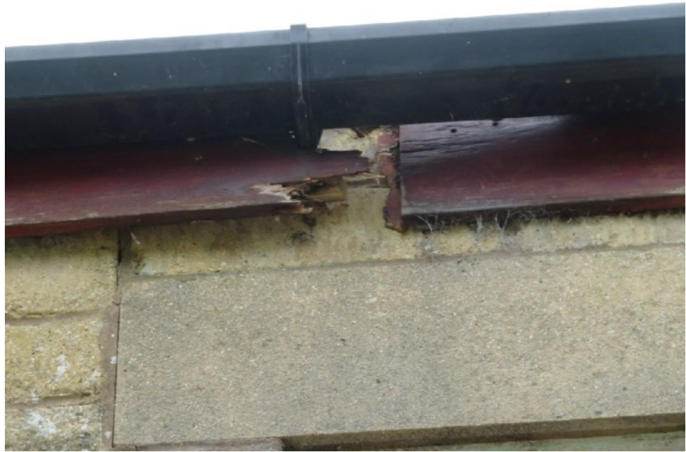
Broken and rotten fascia
