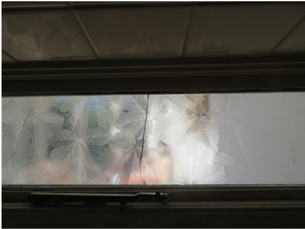
Broken window pane
