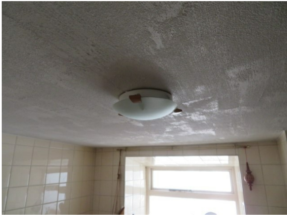
None compliant light fitting
