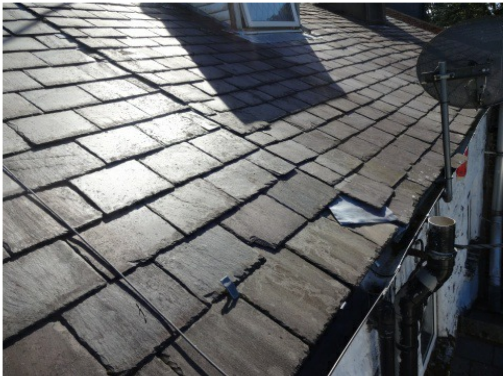
Lack of bird cage to waste stack
