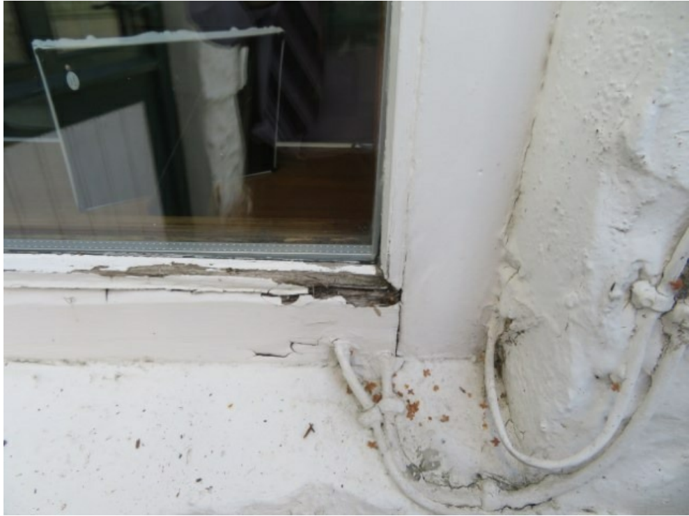
Rot to window frame
