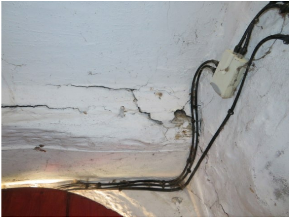
Failed render in ginnell
