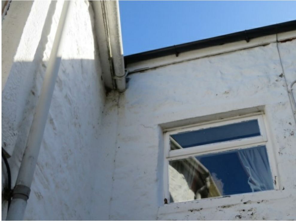
Possible leak to end of gutter
