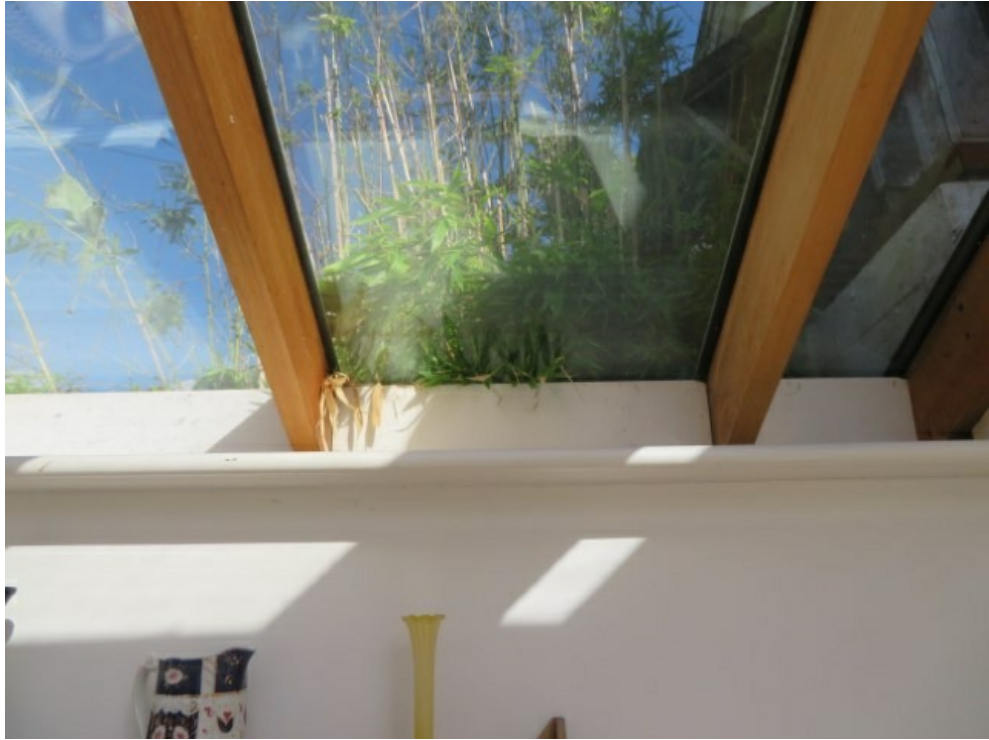
Vegetation growth in conservatory from neighbours property
