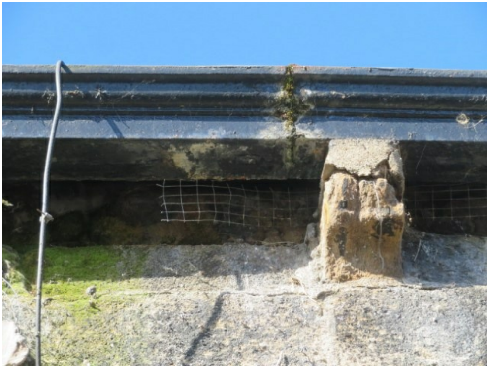
Lack of mesh protection from pests
