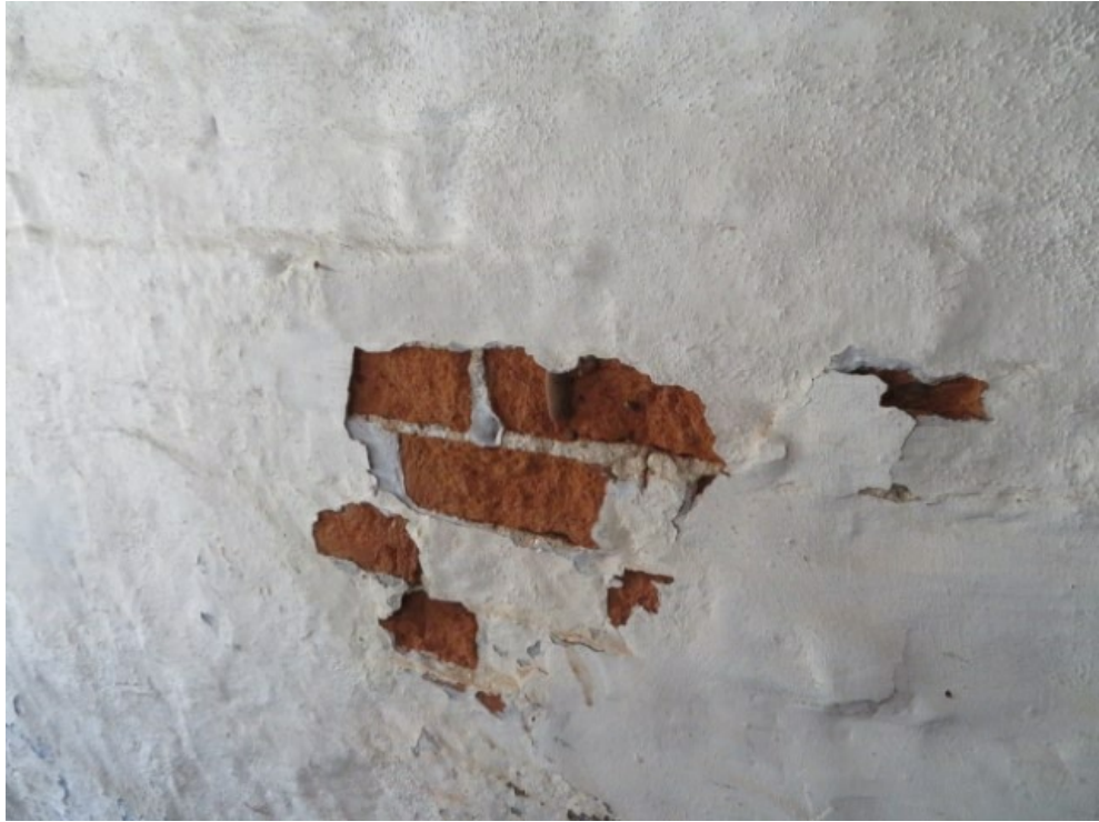
Failed render in ginnell
