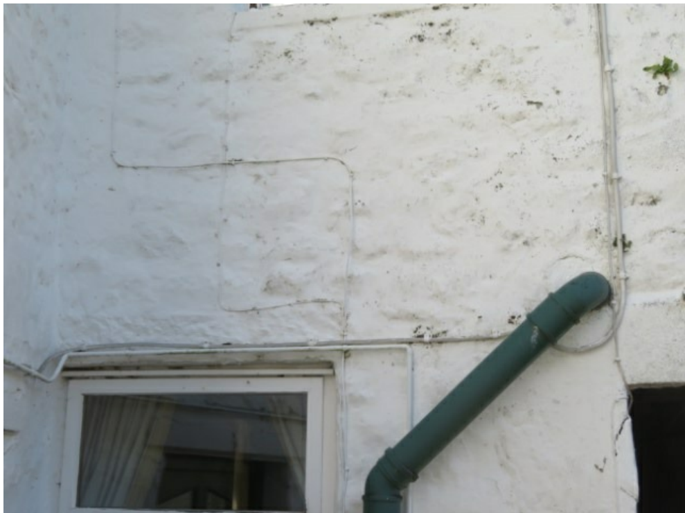
Black stains suggesting damp behind render
