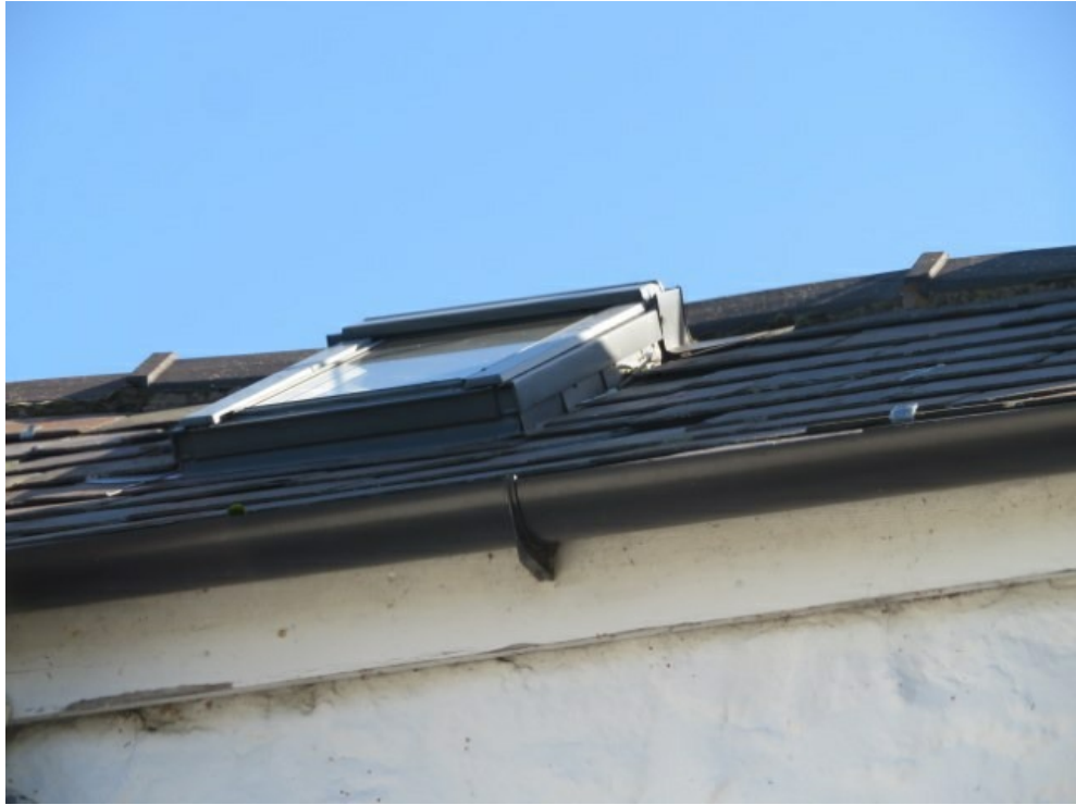
Incomplete mortar to ridge tiles
