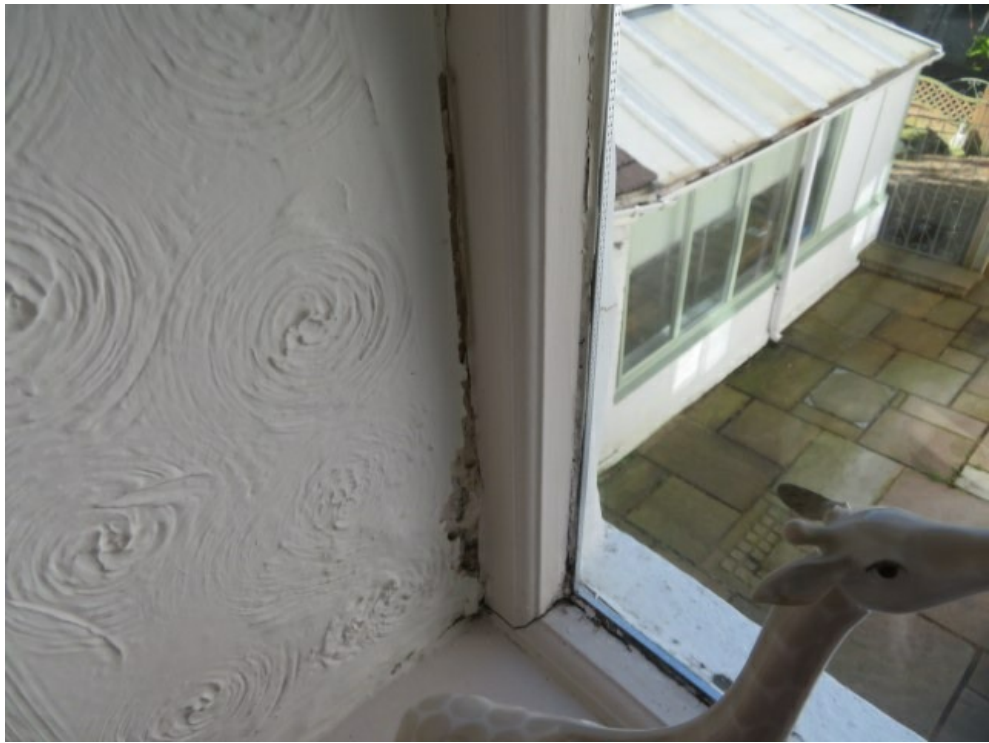
Damp damage to window reveal
