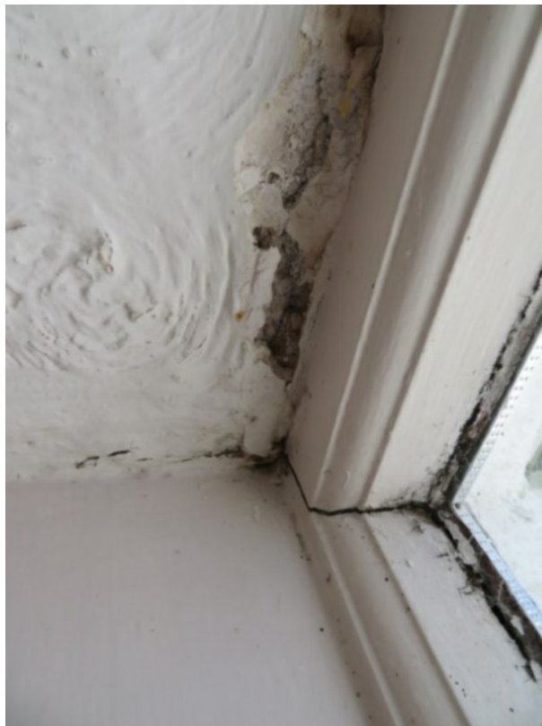
Damp damage to window reveal
