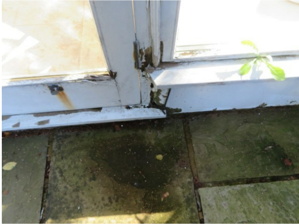
Rot to timber frame and door
