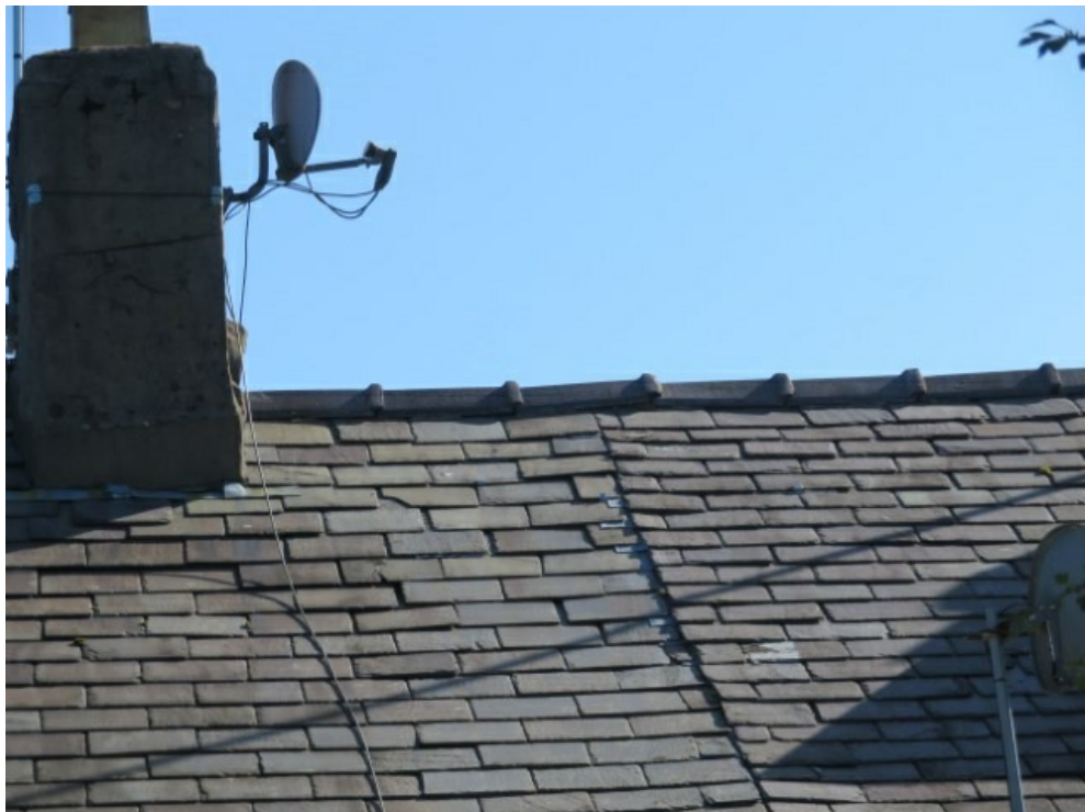
Poor roof junction
