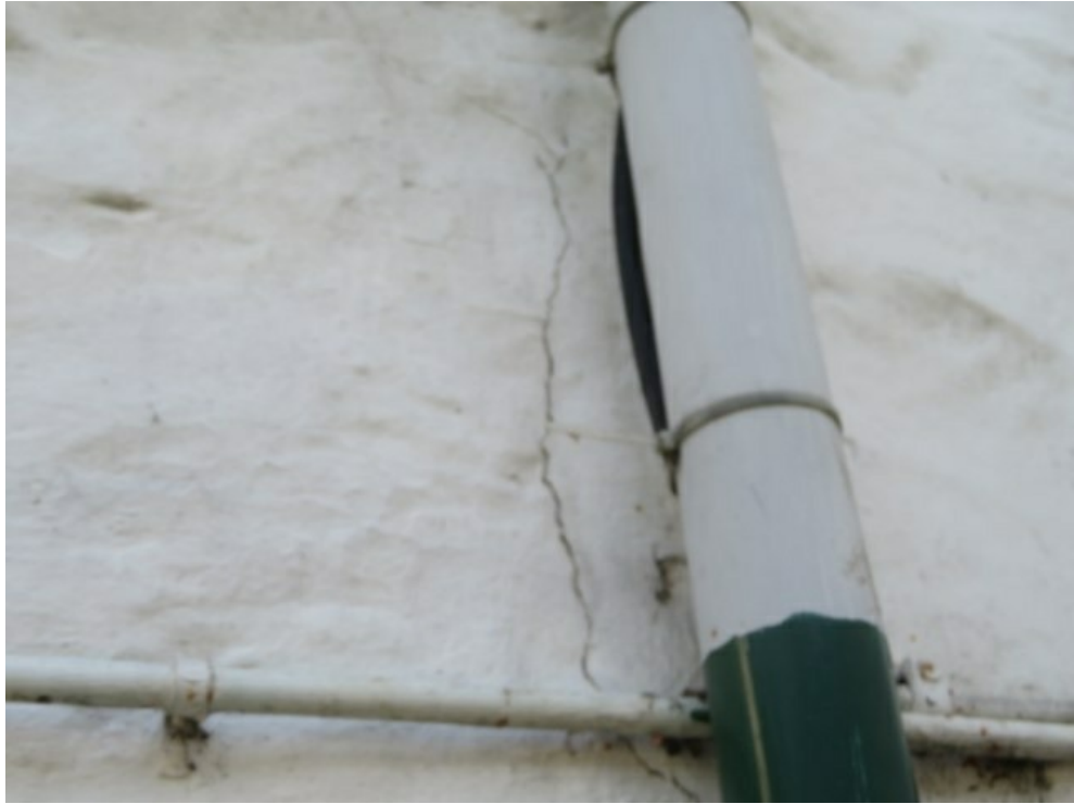
Cracks to render
