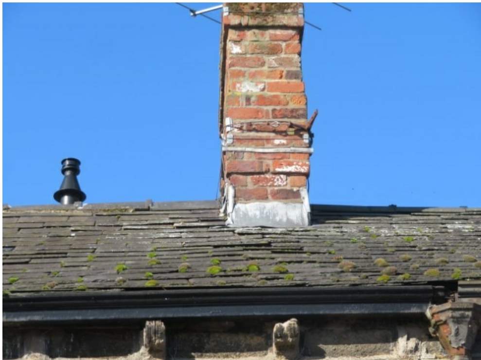
Incomplete mortar to ridge tiles
