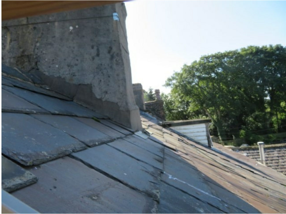
Lack of lead flashing
