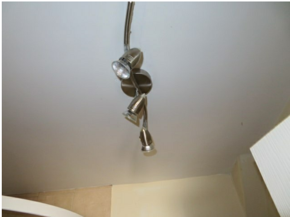
None compliant light fitting
