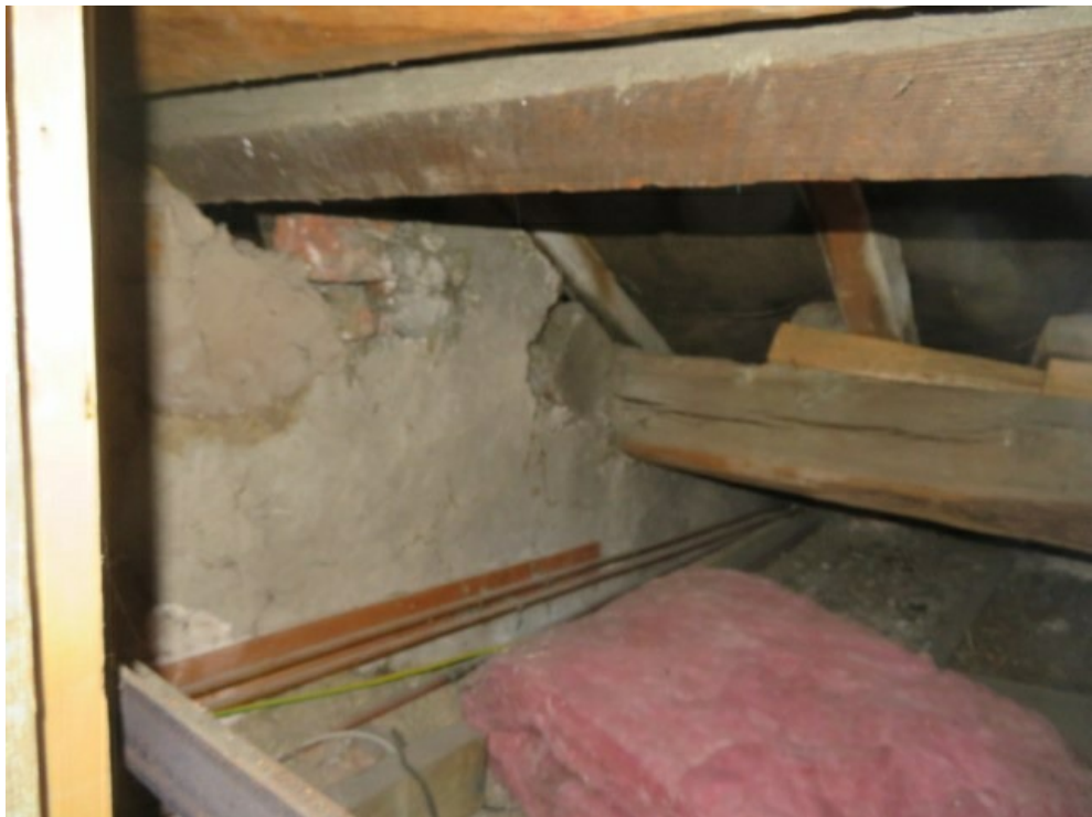
Lack of fire break
