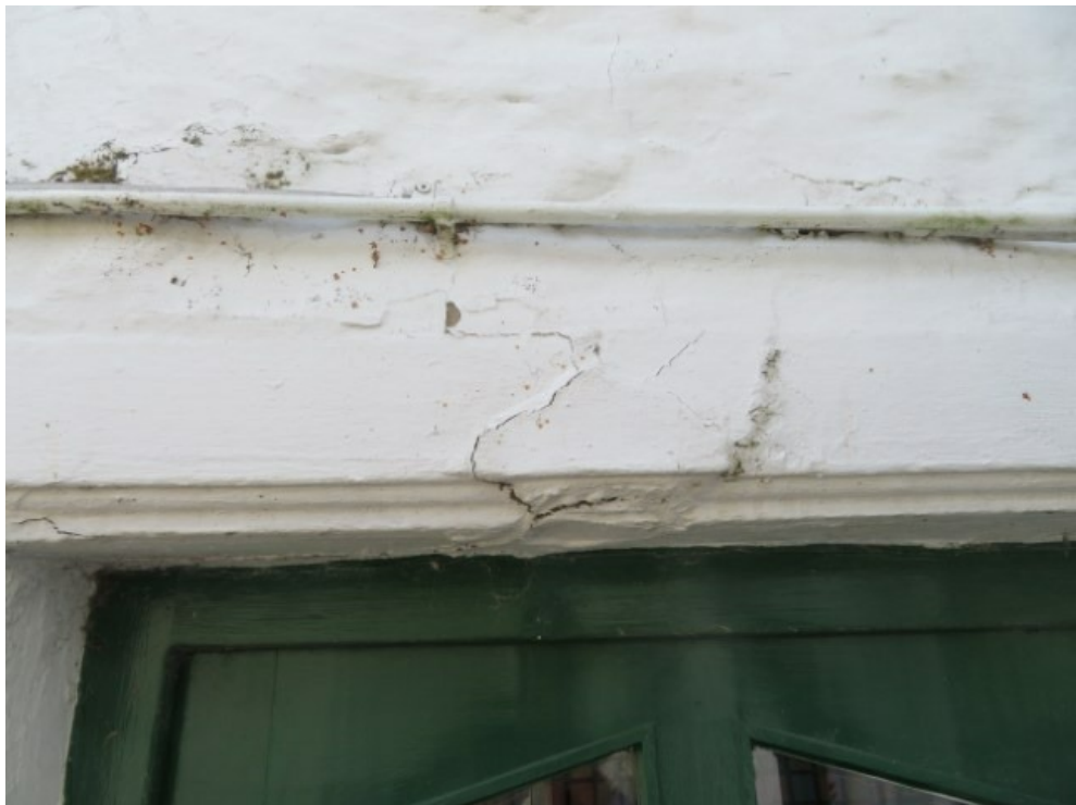
Cracks to render
