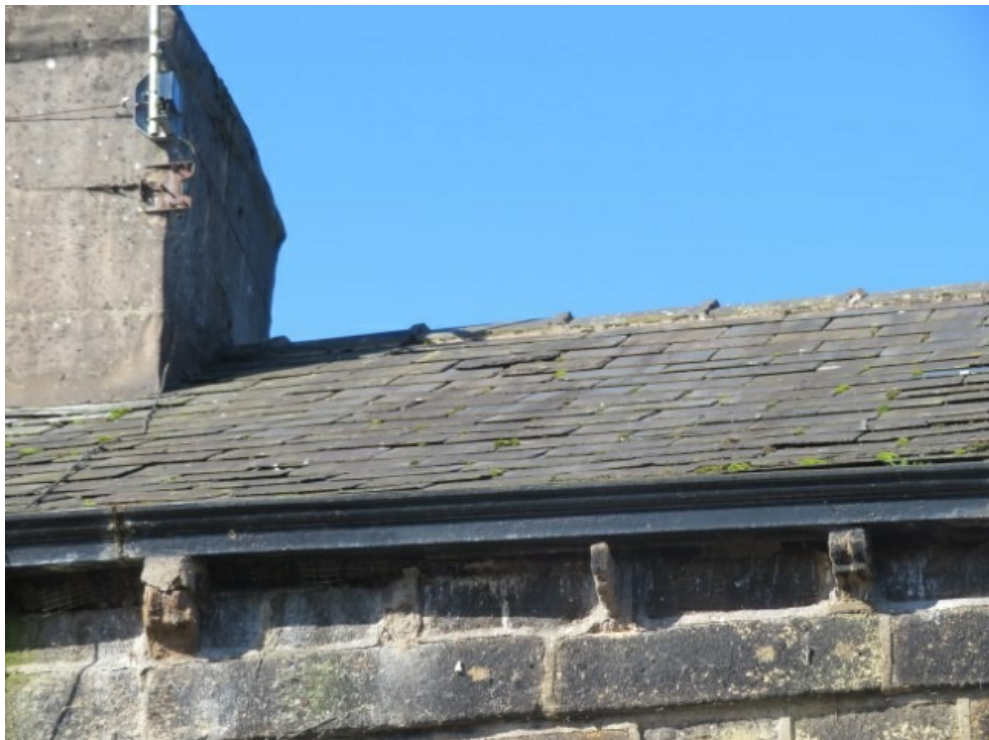
Eroded stone gutter supports
