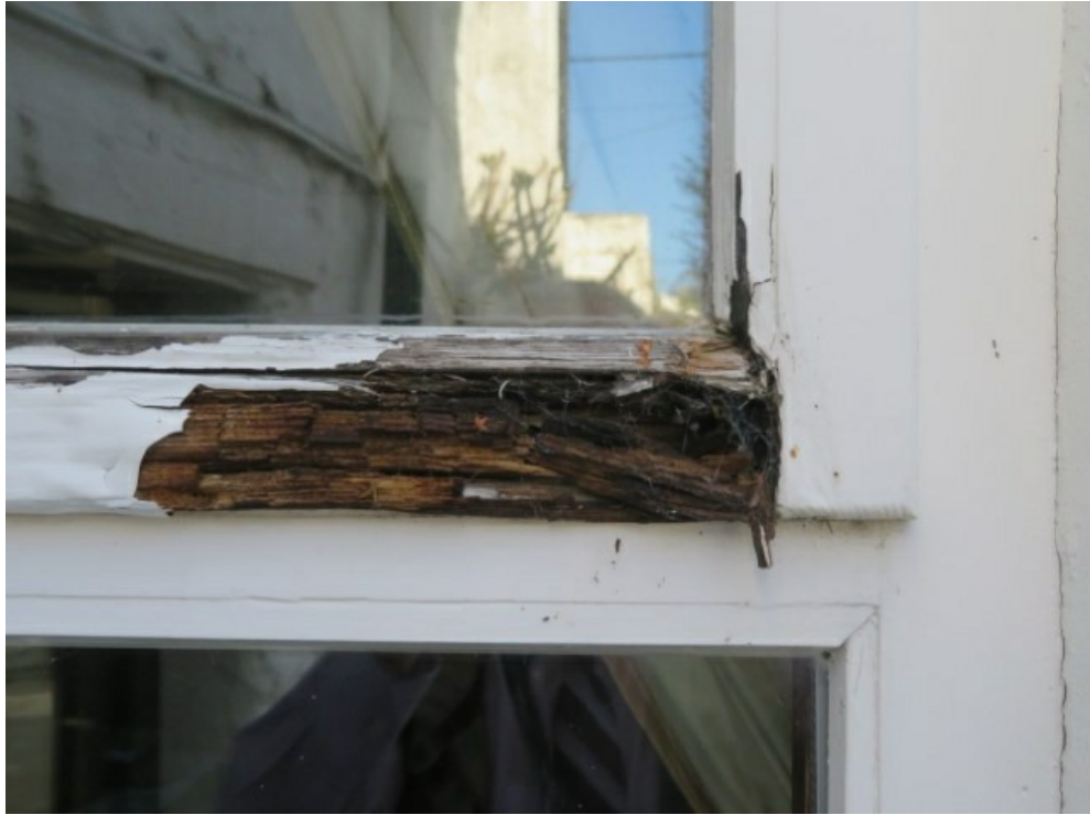
Rot to window frame
