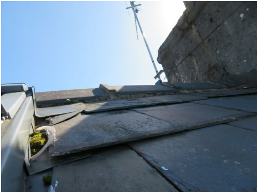
Moss stopping rain run off
