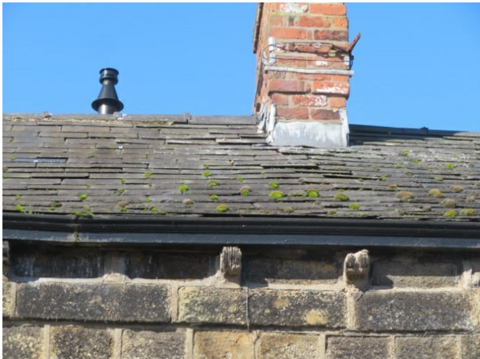
Missing stone gutter support
