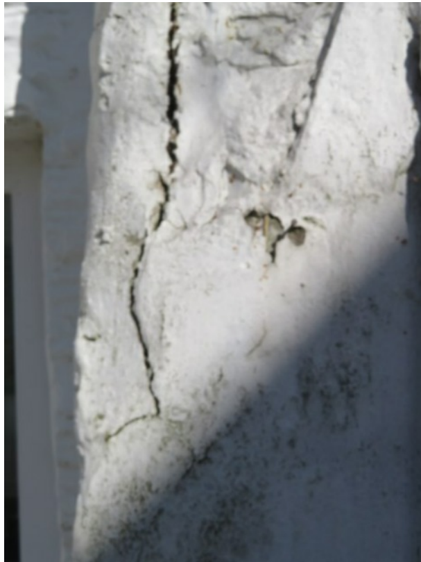
Cracks to render
