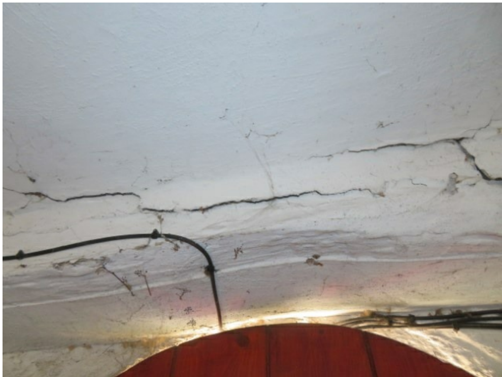
Failed render in ginnell
