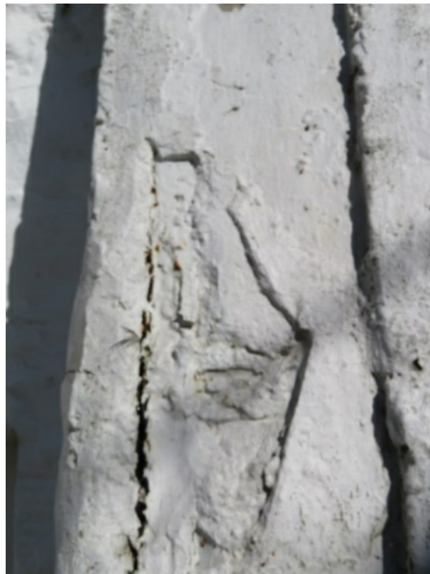
Cracks to buttress
