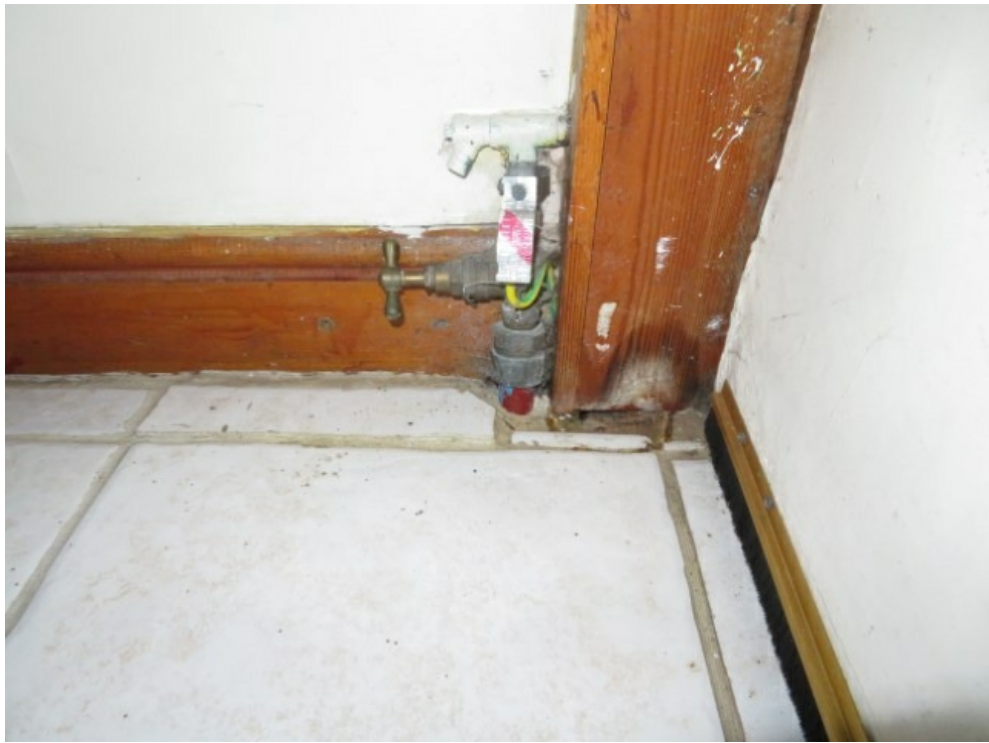
Water stop tap
