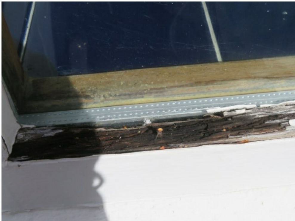
Rot to window frame
