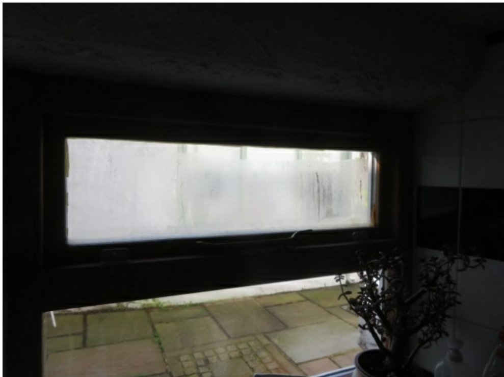
Misted (failed seal) window
