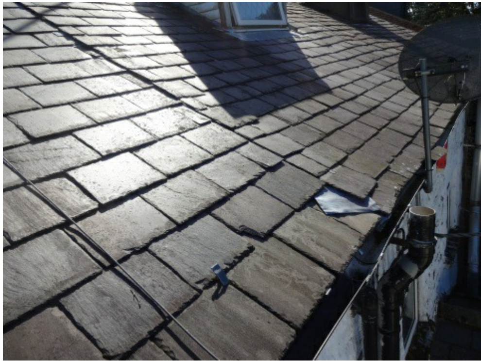
Slipped lead flashing
